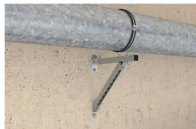
Spiral airduct on cantilever
